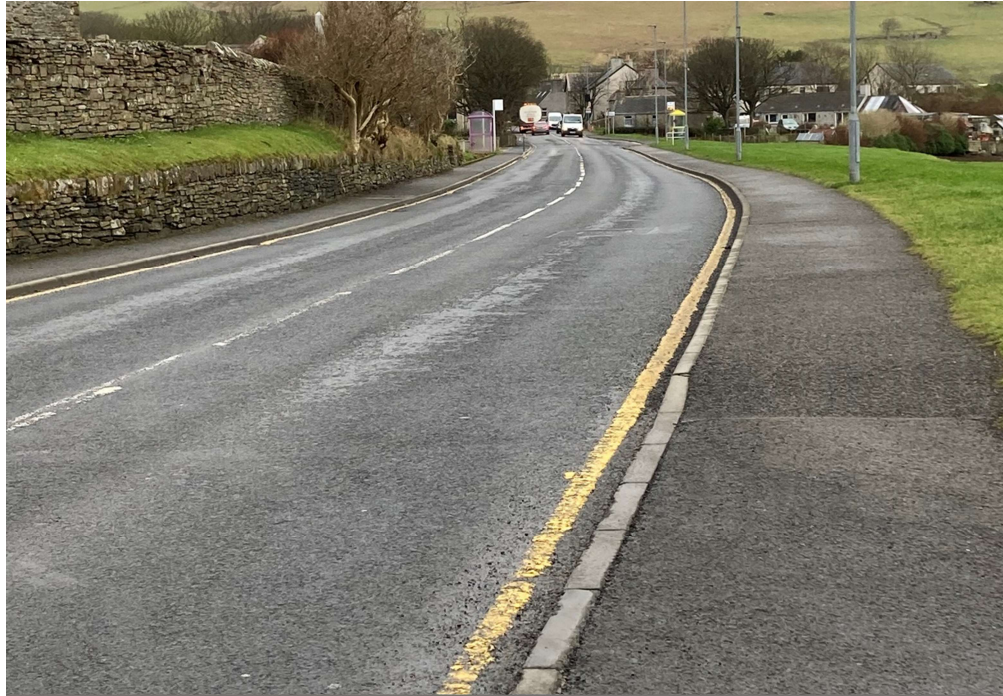
Figure 2. General Standard of Footways on A965
