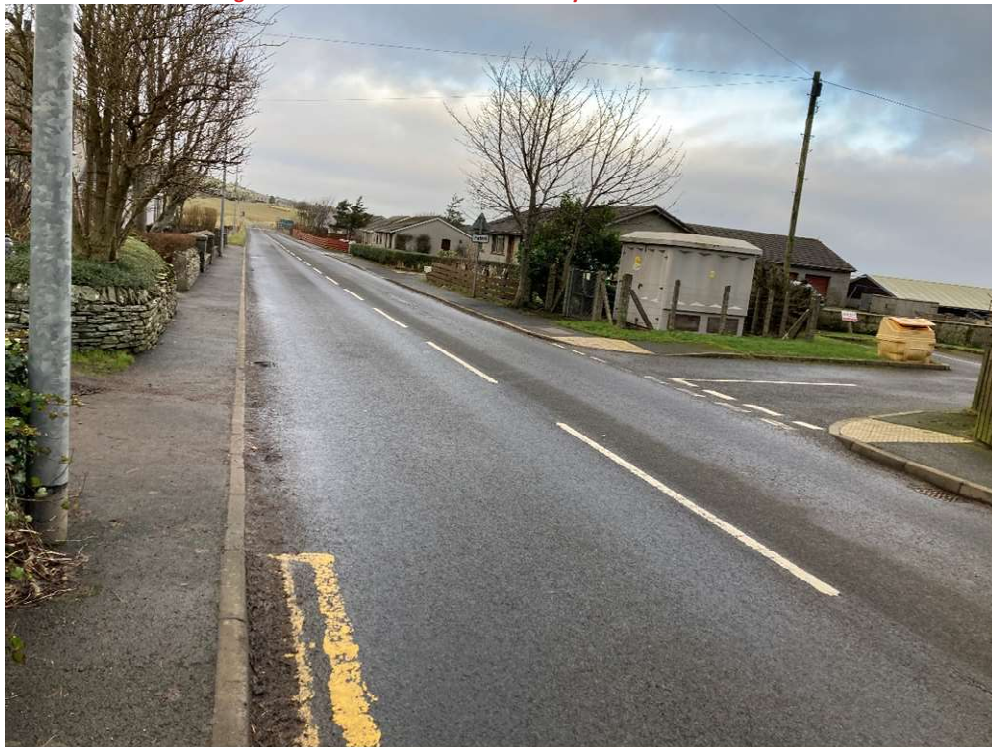
Figure 9. General Standard of Footways on A966
