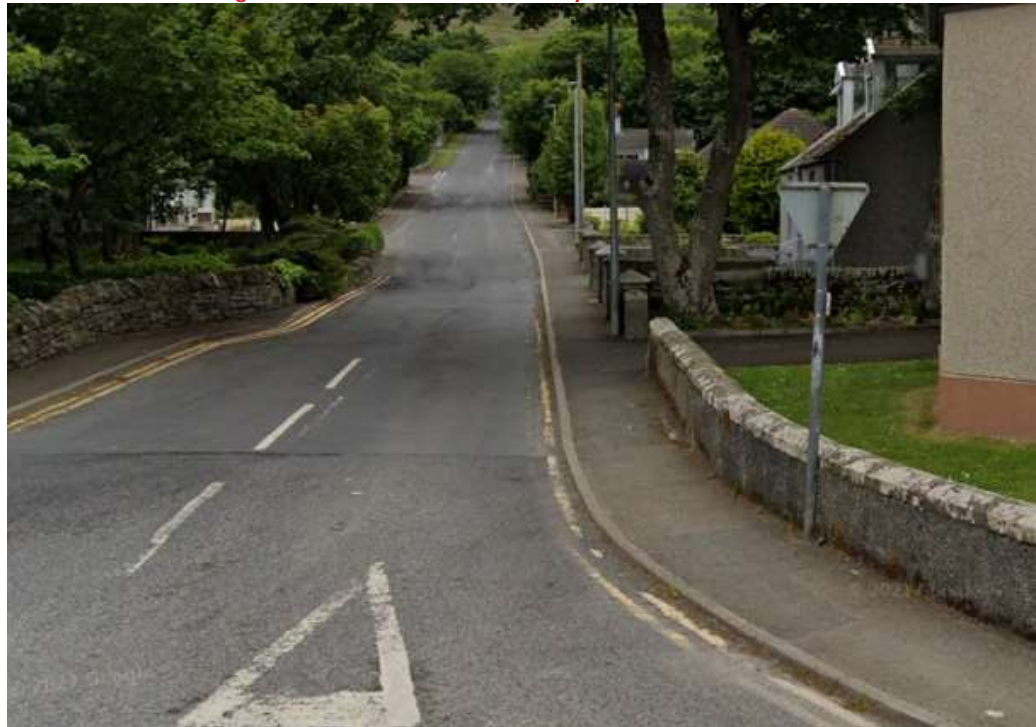
Figure 7. General Standard of Footways on Heddle Road
