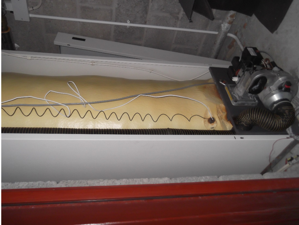
Existing heating system.
