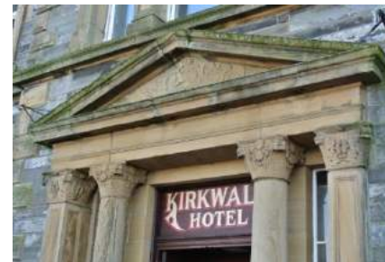
Eroding sandstone on the Kirkwall Hotel
