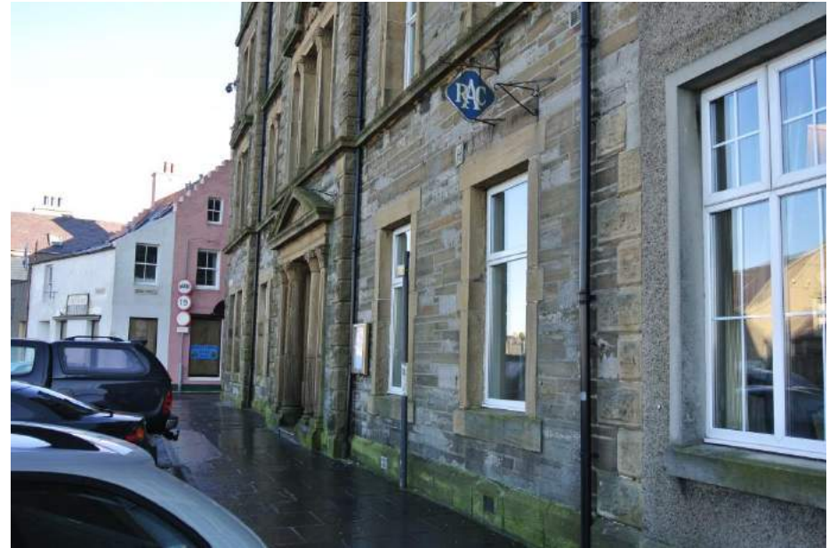
Unsympathetic window replacement at the Kirkwall Hotel
