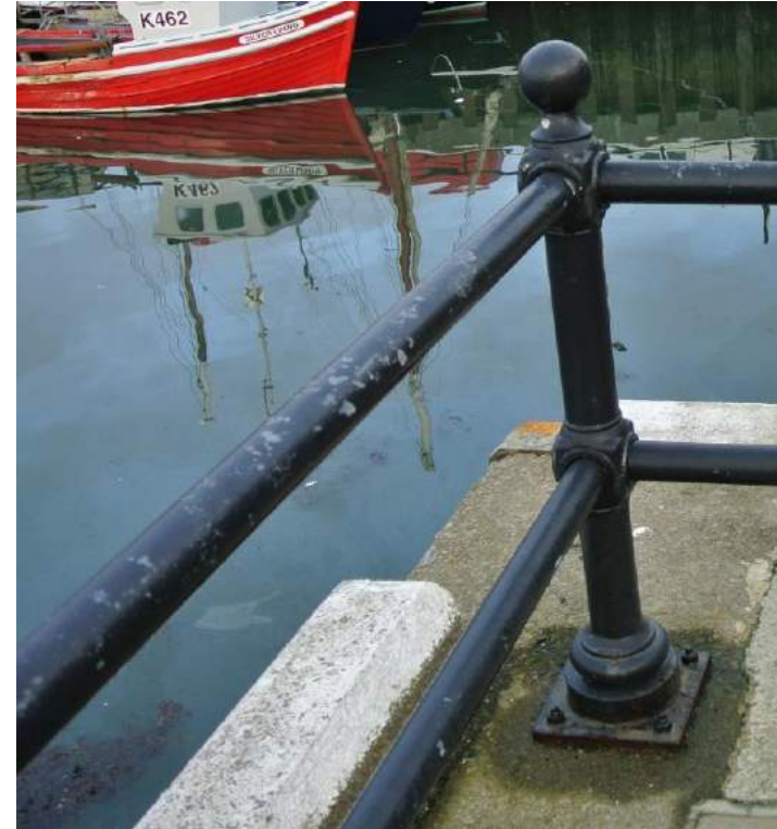
Chipped paintwork on the harbour railings
