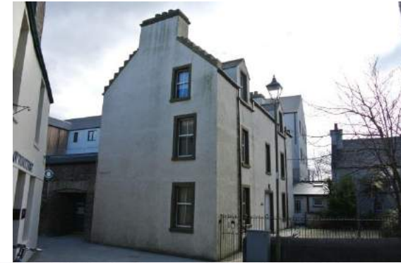
Below: Notes on how 9 Mounthoolie Place contributes to the special character of the area
