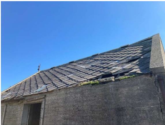
Building 3 holed roof
