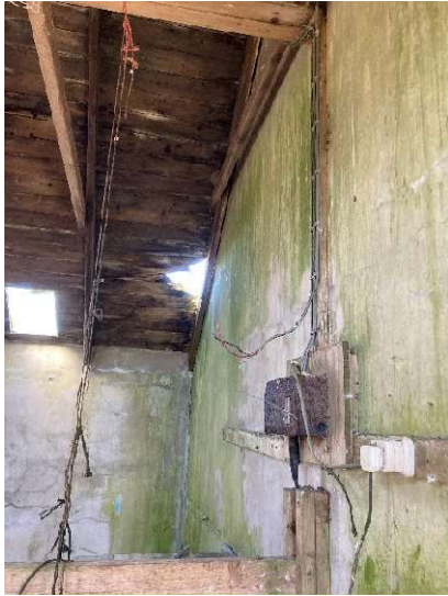
Building 3 interior disfunctional electrics
