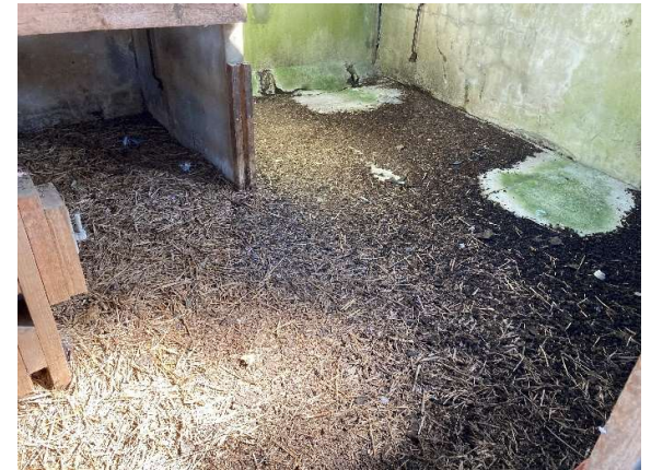
Building 3 interior detritus accumulated over seasons with leaking puddle marks on floor from holed roof
