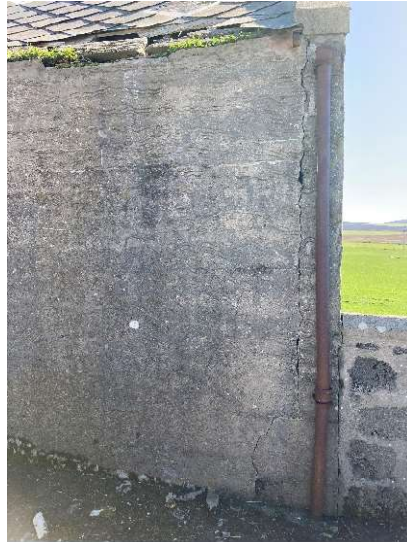
Building 3 cracked render and broken guttering
