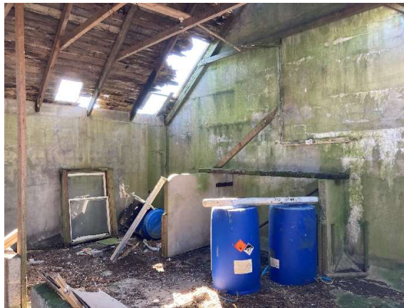
Building 3 interior holed roof
