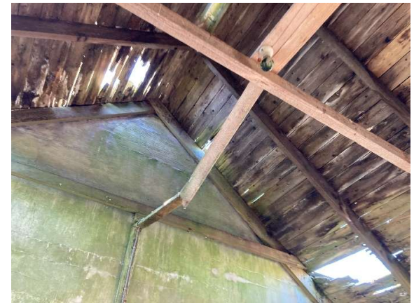
Building 3 interior broken timber roof struts
