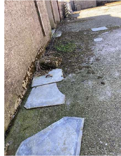
Building 3 fallen tiling
