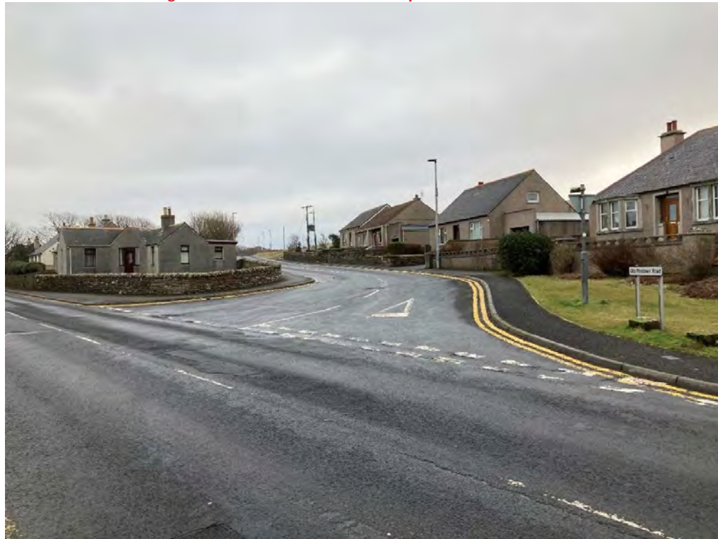
Figure 6. General Standard of Footways on Old Finstown Road
