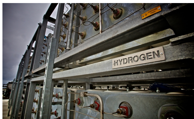
Hydrogen infrastructure in Orkney. (Credit: Colin Keldie).
