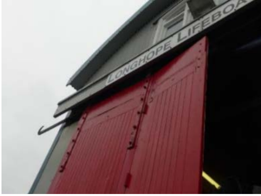
Damaged door hangers
