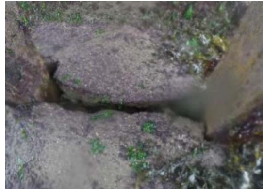
Split in concrete base
