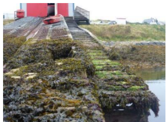
Missing steel floor gantry and rotten western platform
